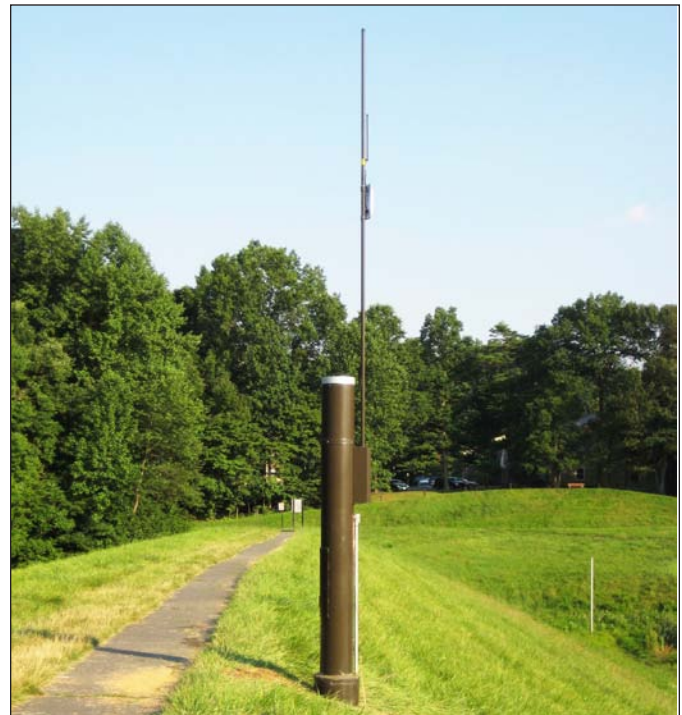
Gauge installed in Fairfax.
