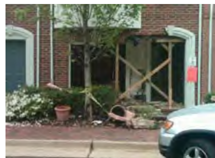
The damaged townhouse on Medlock Lane
