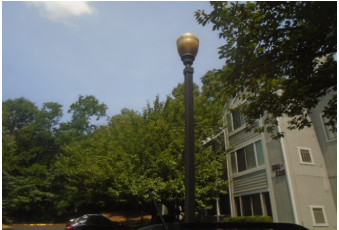
Entry for street lights considers poles, wiring, fixtures and controls will be repaired as needed. No assumption all units will need to be replaced at the same time.
