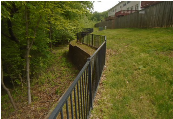
Masonry retaining walls are a "life-of-the property" component-no allowance for total replacement, only spot repairs. Major failure would be catastrophic. Metal railing replacement is a reserve component.
