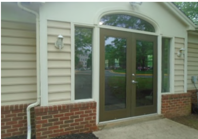
Windows and doors will need replacement when they fail or deteriorated.
