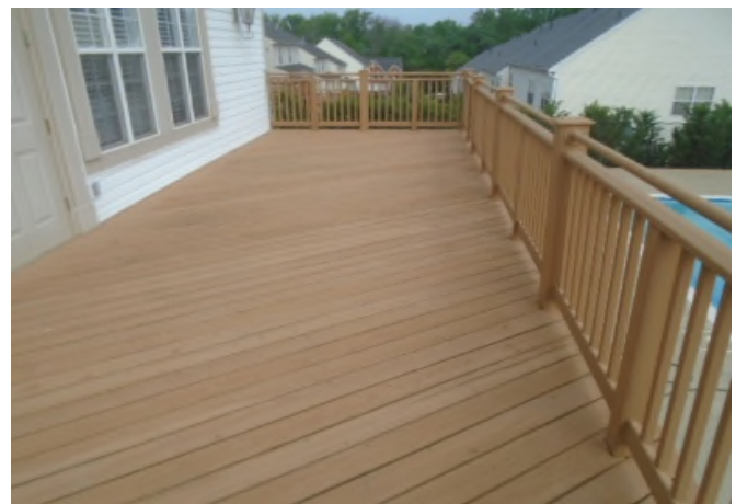
When decks are replaced composite materials should be used. Composites have a longer useful life and require far less maintenance.
