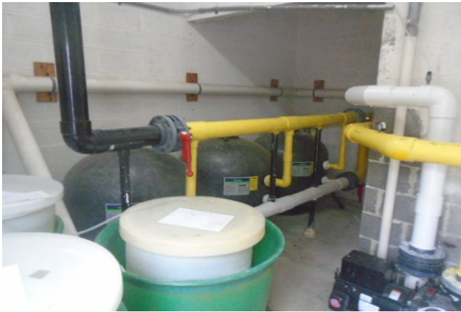
Reserve provides for pool filters, water supply/return piping, chemical treatment equipment and other system components.
