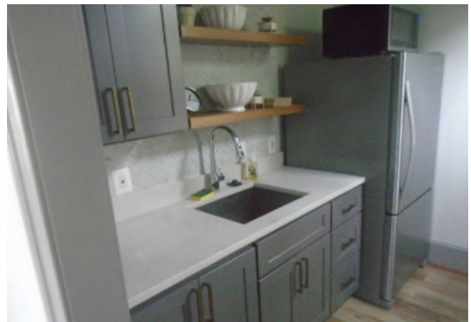
Kitchen is in fair condition; all kitchens eventually need to be updated.
