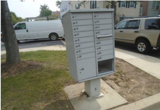
Mailbox replacement will be needed as doors, locks, hinges and other failures occur.
