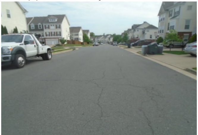
Pavement condition is fair to good. See our recommendations in the "Comments" section for proper care of asphalt pavements. Well maintained pavement enhances property appearance.
